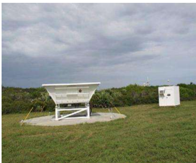
Figure 13. A 915-MHz DRWP at the ER.
