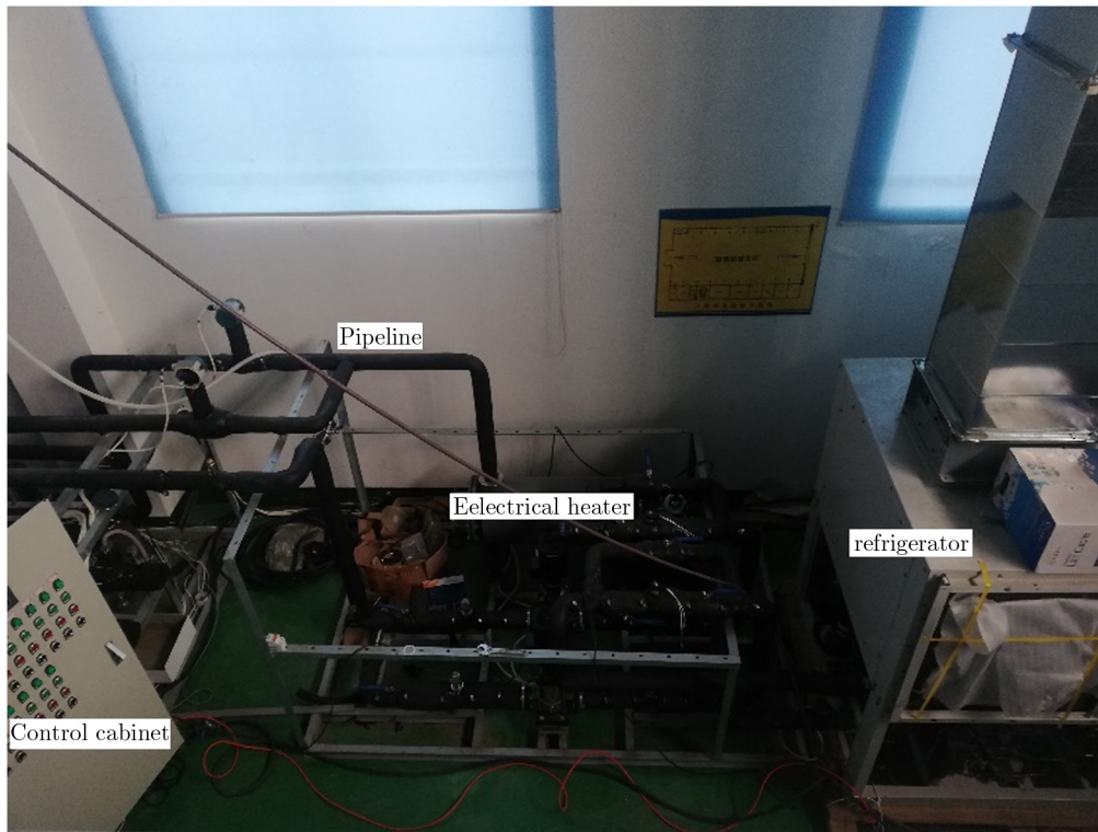
Fig. 8 Experimental device of active temperature control system for CLST.
